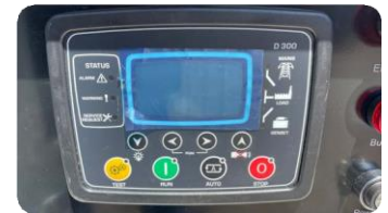
PANEL DE CONTROL
